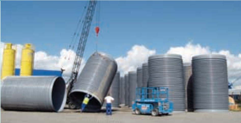
The pipe lengths raised into the vertical position prior to filling the profile with liquid concrete
