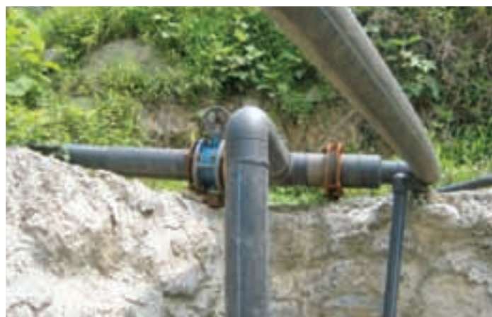
The 160mm PE100 pipe still bringing water from the reservoir to the temporary village of Shengli
