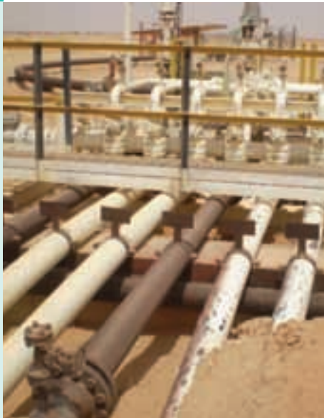
Some of the PE100 pipelines after 15 years operation in the Sim Sim oil field in Oman
