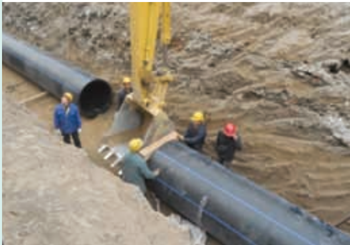
Manoeuvring the 1200mm diameter pipes into position for the LiangMaiQiao water recycling project
