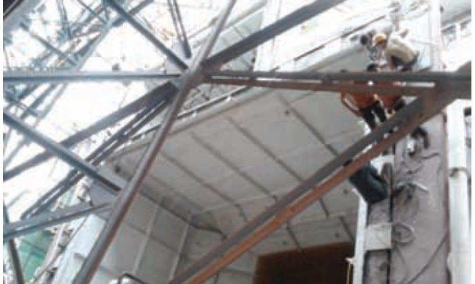
A "bird's eye view" of one of the large process tanks lined with BorECO PP sheets
