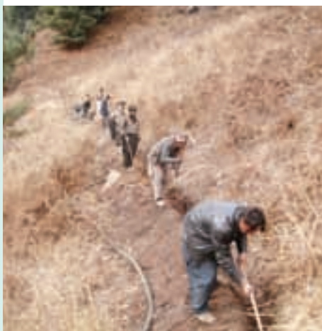
Villagers installing the PE pipe in the trench down the steep mountain side during the first project
