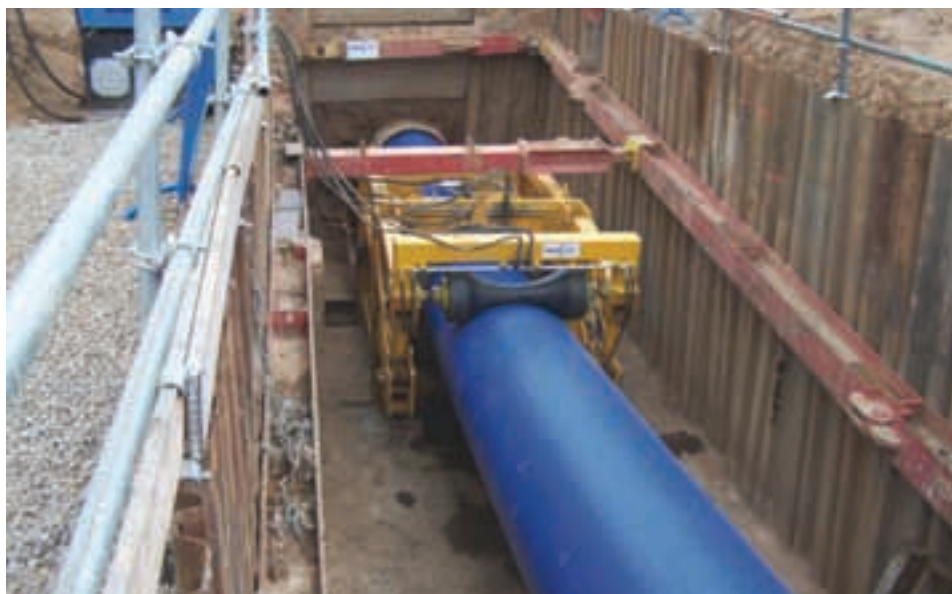
The Swagelining of an old 39 inch cast iron water main with a 1016mm PE100 pipe in the UK
