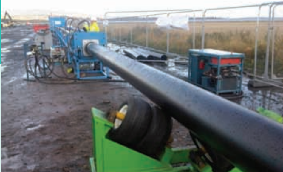
Installation of a PE100 liner into a riser for subsea service in West Africa
